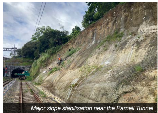
Underslip on the Eastern Line
