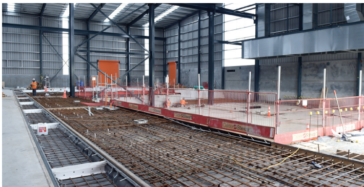
Interior of mechanical building (photo courtesy of Otago Daily Times).
