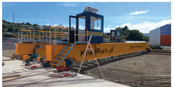
The traverser beams and cab have arrived on site, painted Otago blue and gold colours.
