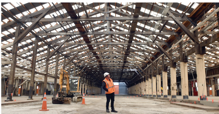
The oldest building onsite, known as the machine shop and built around the 1870s, has been strengthened and repurposed.
