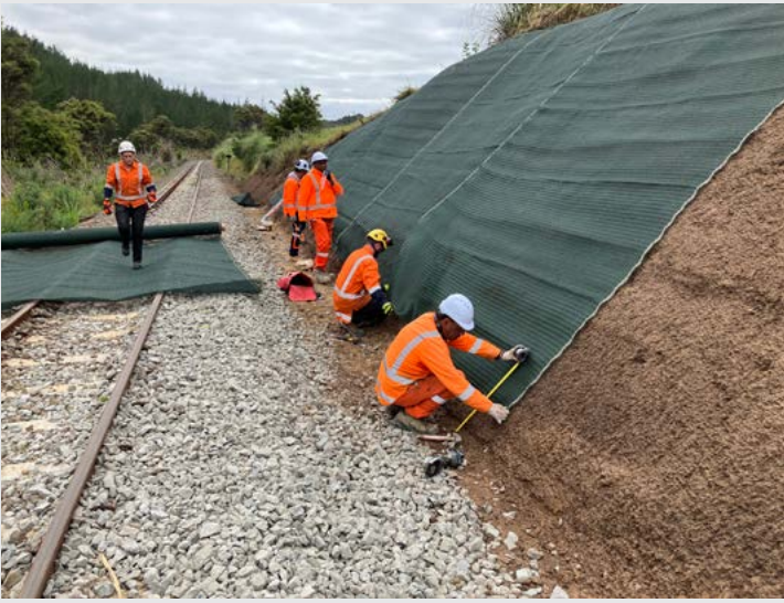
Stabilising mesh being added to a cleared embankment beside the track near Topuni.
