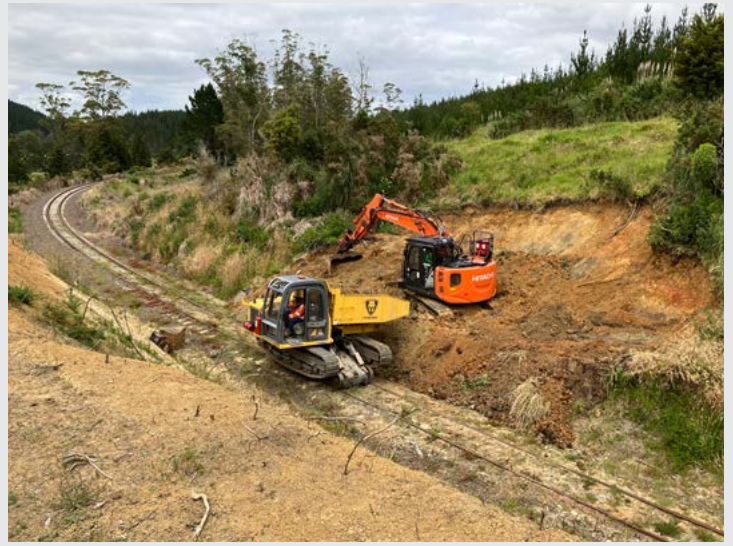
Another slip being cleared near Topuni.
