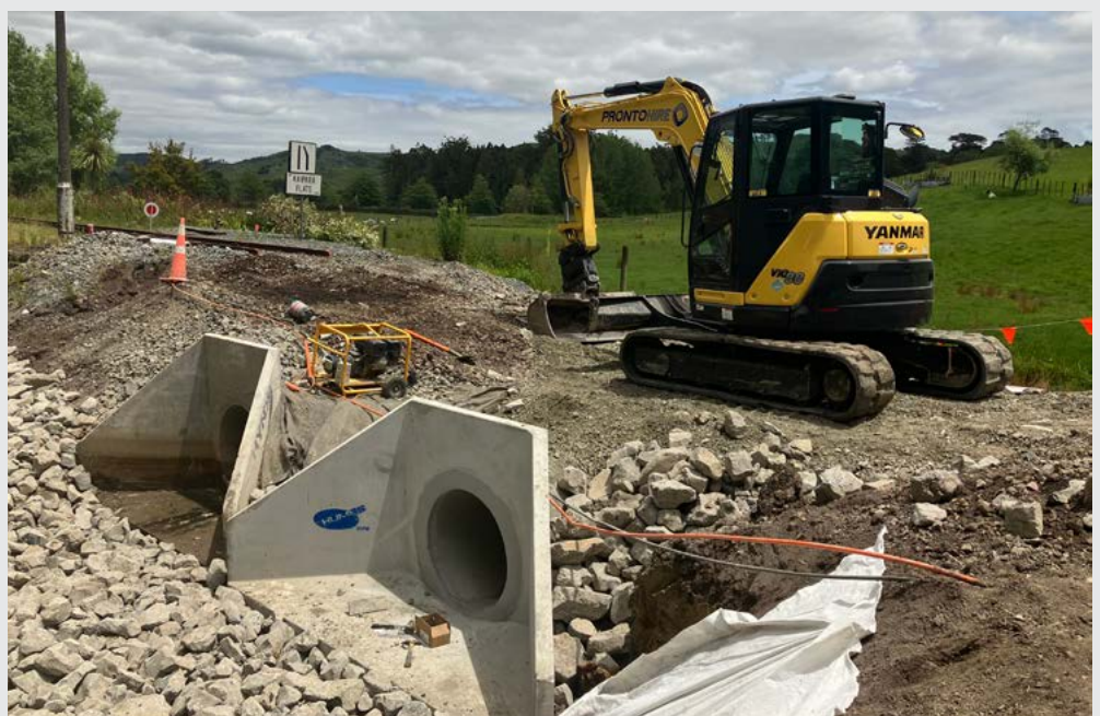
New culverts, to improve water flows, being installed under the rail line in the Kaipara Flats area.
