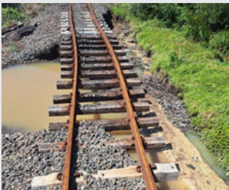
Washout on the NAL
