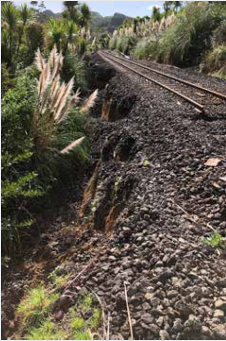
Example of an underslip near Tahekeroa
