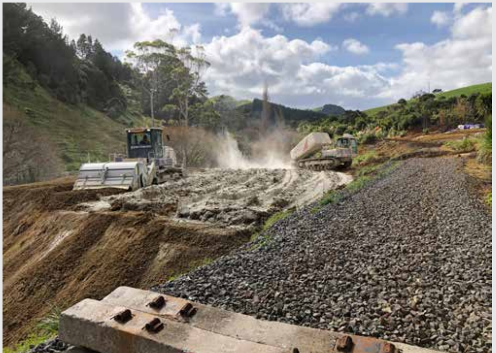
The rail corridor at Tahekeroa has been cleared and landslip material is being stabilised at a temporary fill on site beside it.
