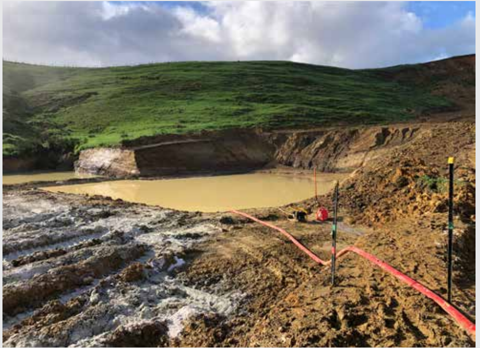
Example of ongoing weather impacts - having to drain water from excavations at Tahekeroa
