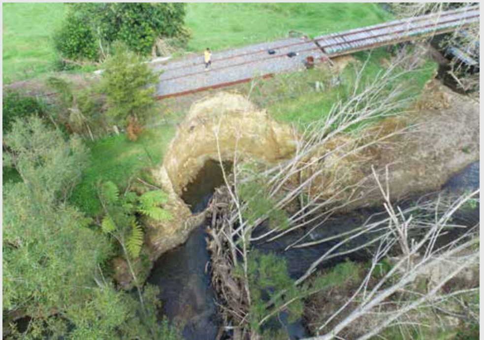
Example of river scour near Whangārei
