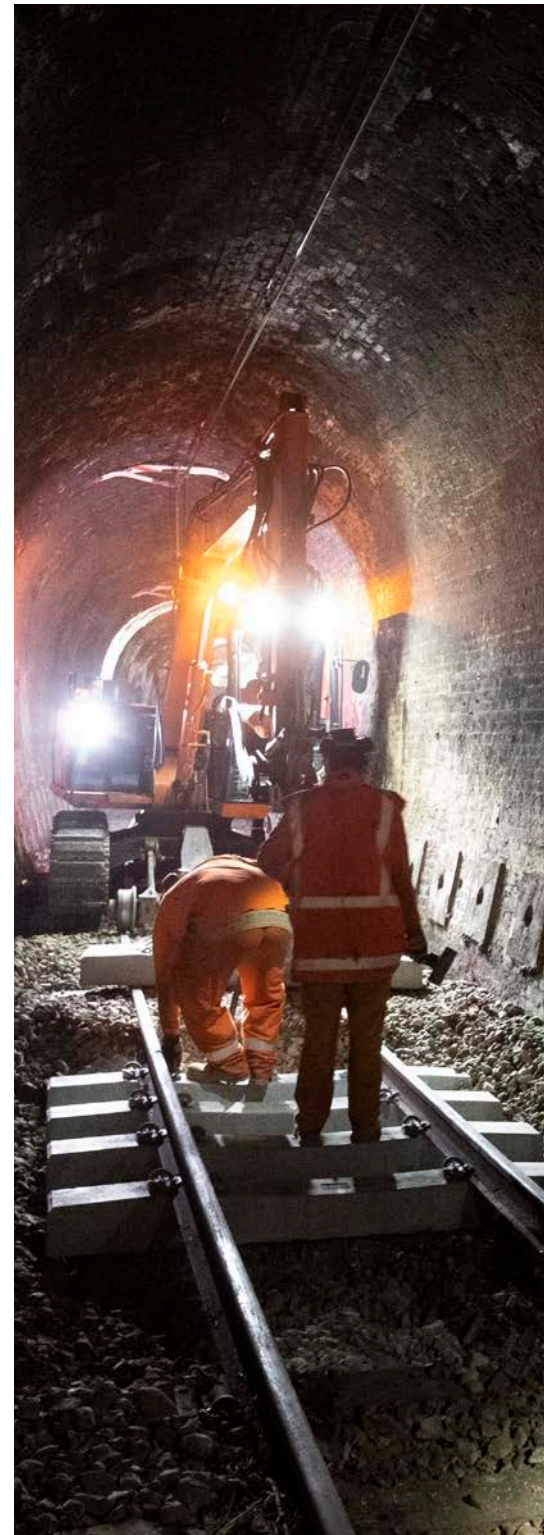
KiwiRail is carrying out extensive upgrades on the Wellington commuter network, including in its tunnels.
